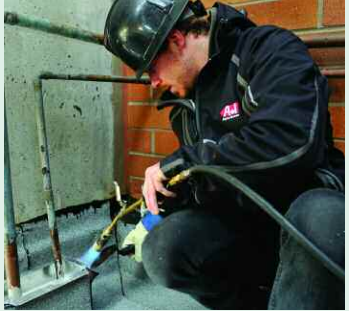
Rofer Aaron Dunn is in a trade that is changing due to the complexity of new roofing materials and applications, more rigorous safety requirements of WorkSafeBC and the concerns of younger workers who don't want to put their lives on the line.
