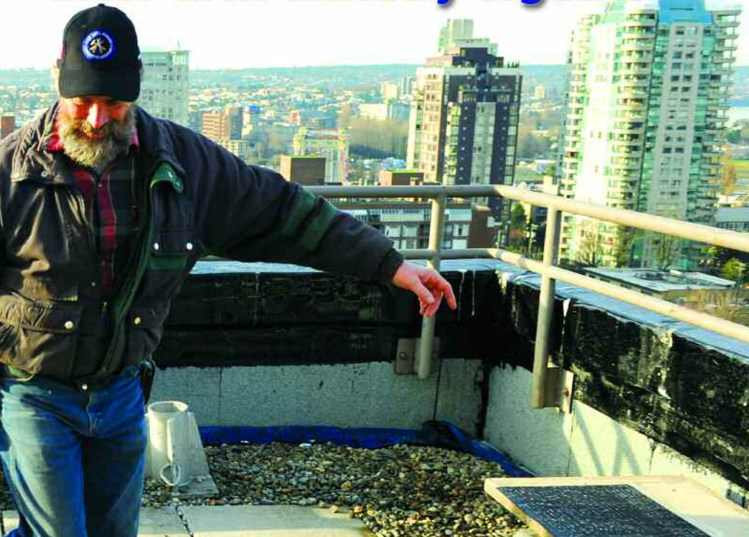
Aaron Dunn and Ron Lacey, members of the Sheet Metal and Roofers Union Local 280, prepare to do torch-on roofing atop a 16-storey building in downtown Vancouver.
