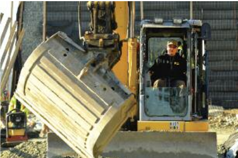
Members of Operating Engineers Local 115, Ironworkers Local 97, and Teamsters Local 213 are also working on the Low Level Road Project.
