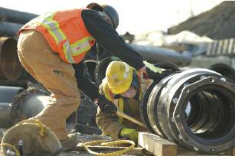
Nick Remillard and Nathan Boon working on the watermain fittings. The pipelines are being replaced, expanded and upsized. "Some of the pipe is really old and too small," Boon said.
